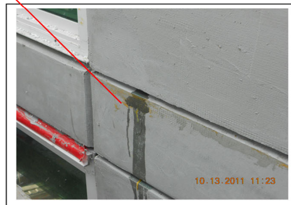
24 6 th floor water at joint below ok
