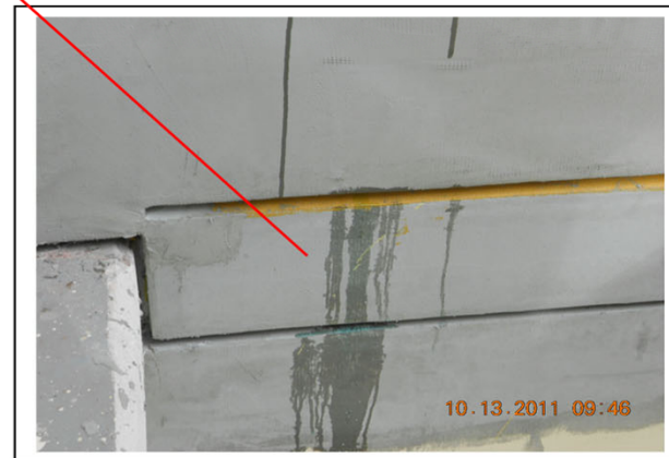
12 4 th floor water at joint below ok
