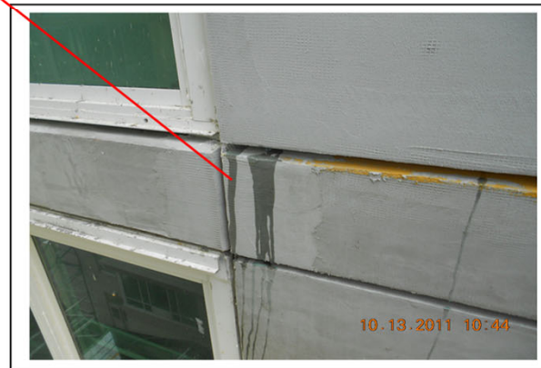
20 6 th floor water at joint below ok
