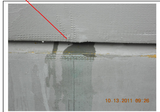
8 8 th floor water at joint below ok
