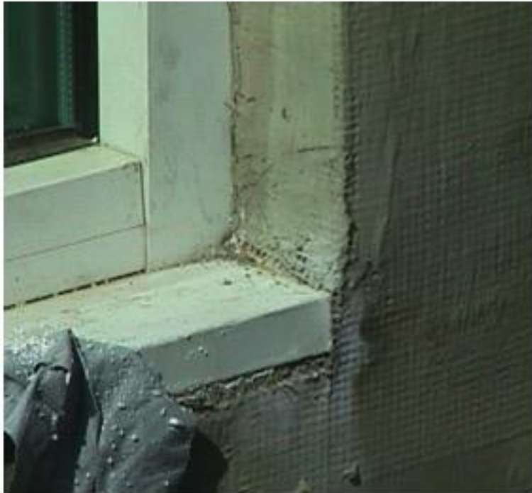
Original sill pan evidences water below sill/jamb corner
